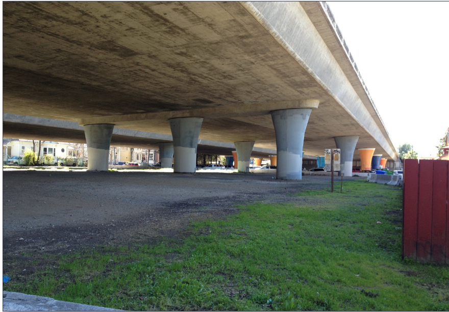
FIGURE 4.9 Strip of open space located on the southern end of the study area
